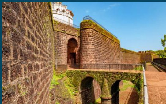
Restoration & Upgradation of Forts Location: Cabo De Rama Proposed Funding : INR 17 Cr
